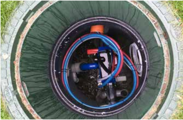
Visual check of the treatment system
