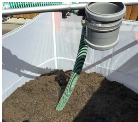
Figure 11: Readjustment of the metering pump, filtration without excess water (under dosing) or foams (overdose)
