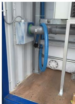
Figure 3: Suction hose for desludging in the container.blue
