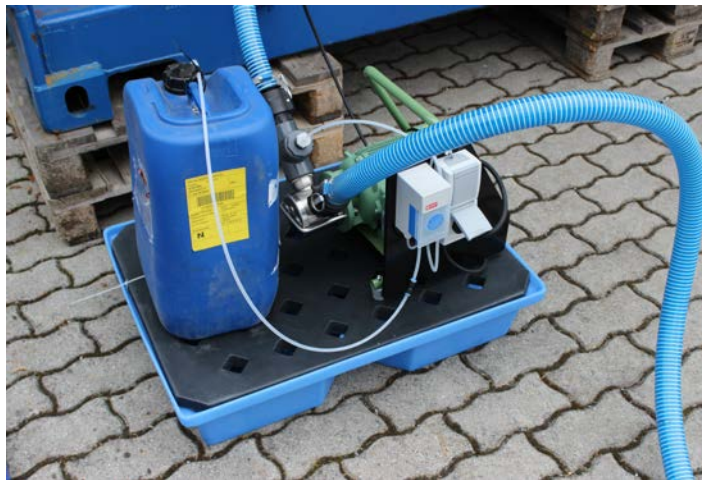
Figure 4: Pump unit with carrier frame next to the flocculant on the drip tray
