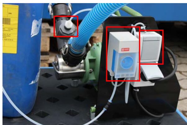
Figure 9: Dosing pump, toggle switch and injection point for the dosage of flocculant
